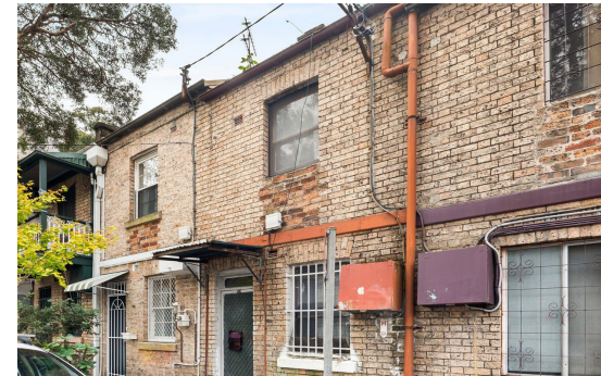
56 Smith Street, Surry Hills before Source: realestate.com.au
